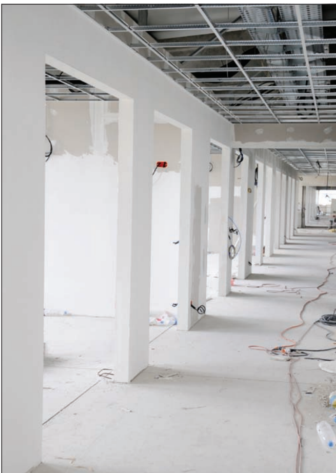
Walls that only partially extend above the ceiling grid incur additional costs and limit flexibility like deck-to-deck construction, while also permitting sound to flank through both the ceiling and plenum like floor-to-ceiling walls.
