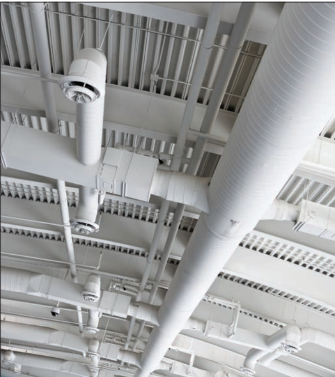
Sealing a wall to the deck is challenging given both obstructions and the prospect of an uneven deck surface.
